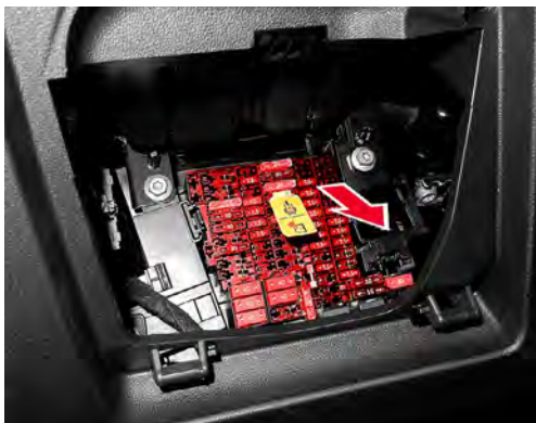
Emergency cut-out connection, fuse carrier
